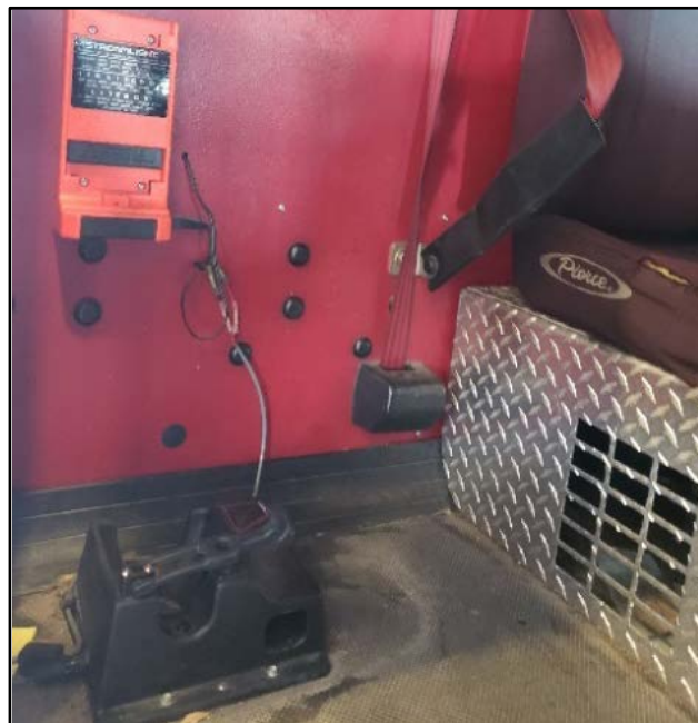
Photo 3. Aerial Platform 1 replacement apparatus. TIC charger bolted on the floor behind the officer’s seat. (Photo courtesy of the fire department.)
