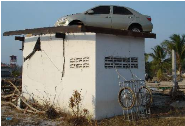
Post-tsunami devastation in Phuket, Thailand.
