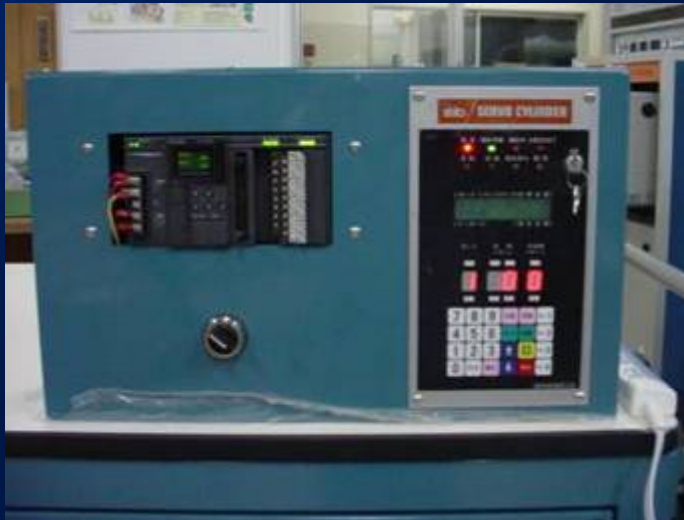
② Control Panel
