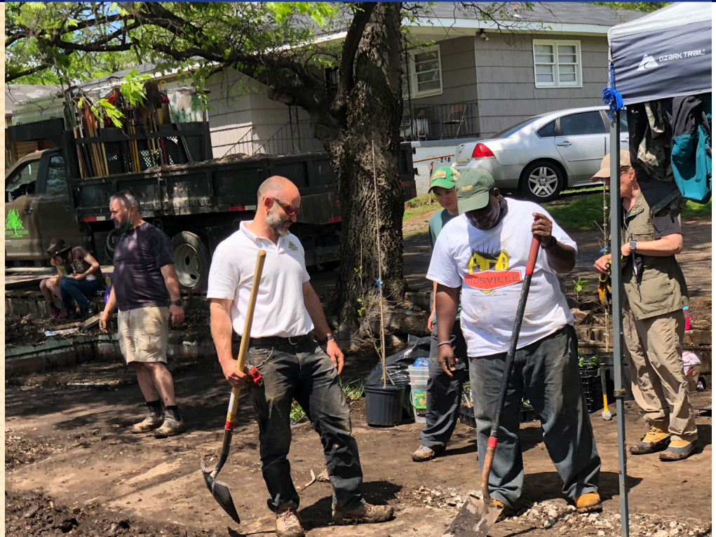
In April 2021, volunteers worked in Titusville's new Triangle Park to plant native species, install picnic tables, and install a gravel path.
