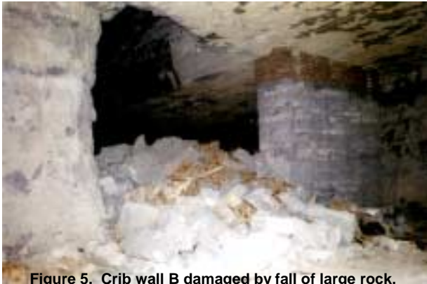
Figure 5. Crib wall B damaged by fall of large rock, October 1996.
