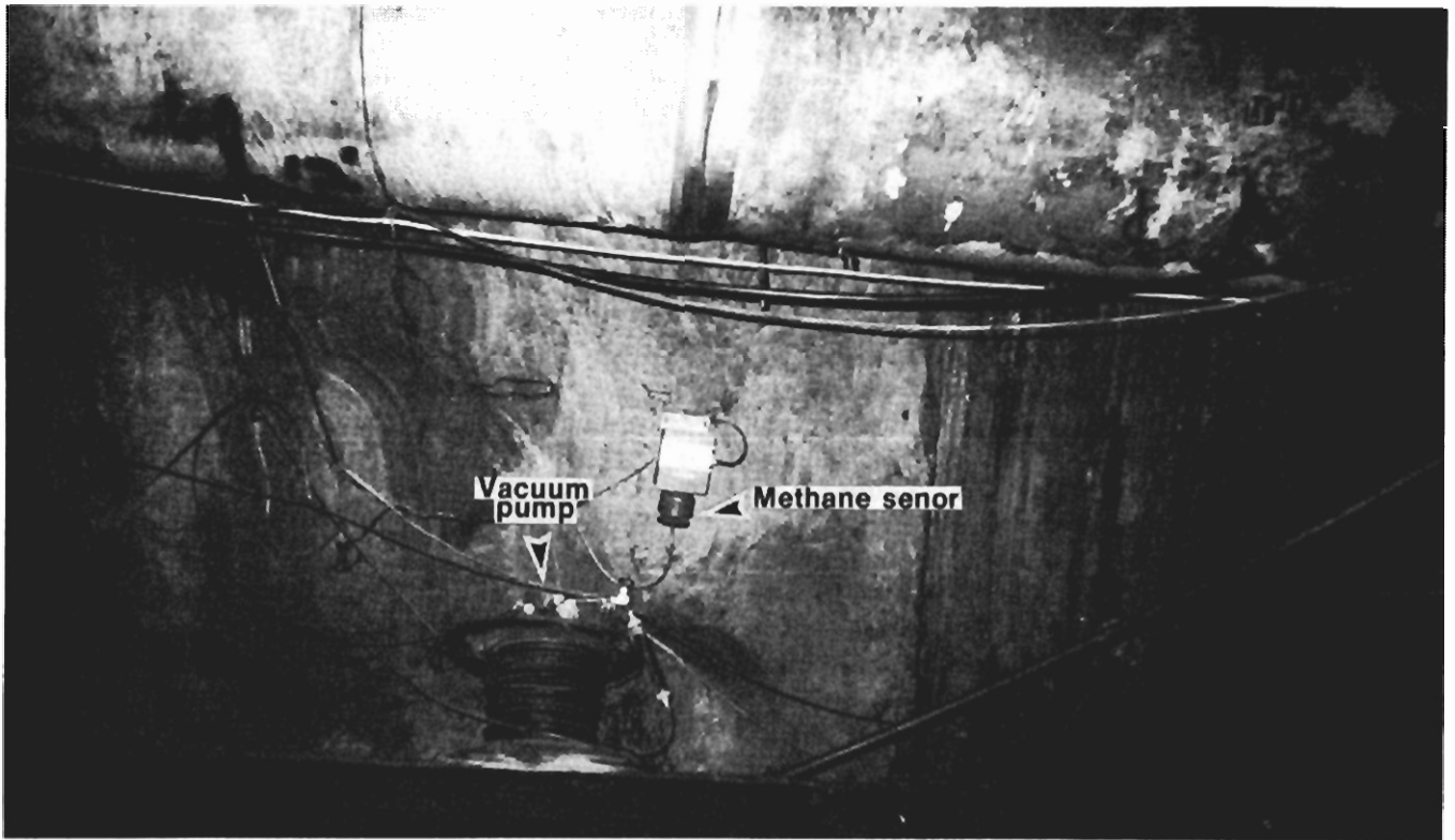
FIGURE 12. - Vacuum pump and methane sensor for collecting and measuring methane concentration in exhaust duct.
