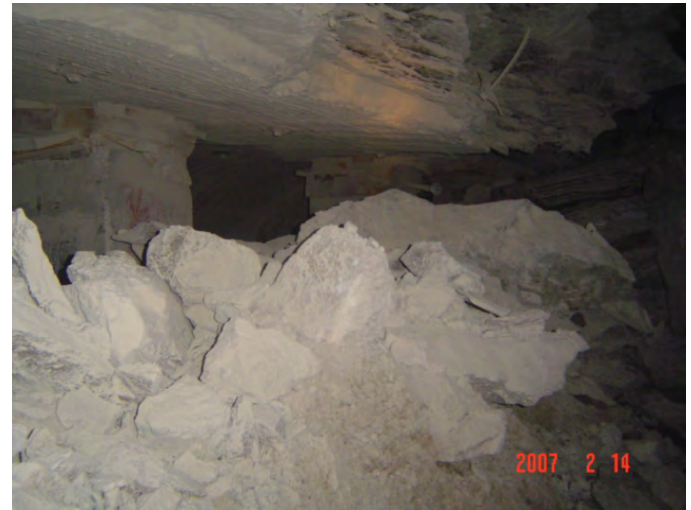
Figure 4. Poor Ground Conditions.
