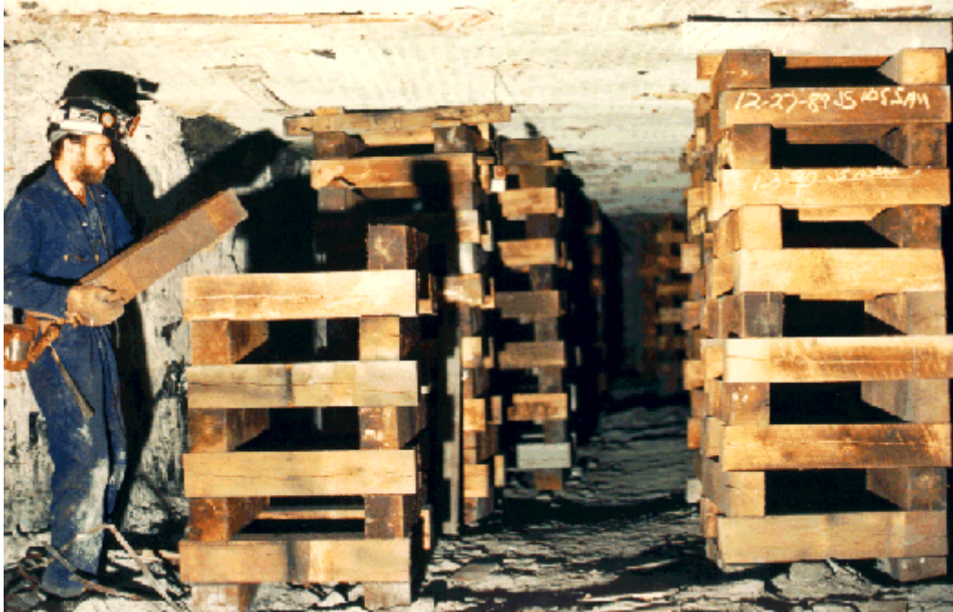
Figure 1.—Installation of cribs in a longwall tailgate entry. (Photo by Frank E. Chase, NIOSH Pittsburgh Research Laboratory.)
