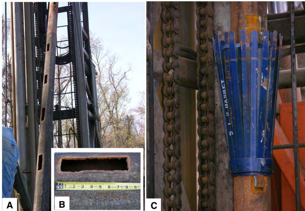
Fig. 2. A pictorial showing of a slotted casing ready to be lowered (A), the dimension of each of the slots (B) and the baskets (C) used above the slotted interval to stop the cement to flow beyond intended interval.
