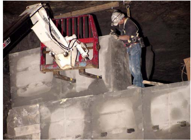
Figure 2. Setting blocks for construction of a Super Stopping using extended reach fork lift and precast lifting holes.
