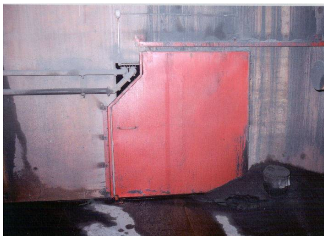
Figure 3b. Seal installed where connecting tunnel accesses main structure in basement of facility.
