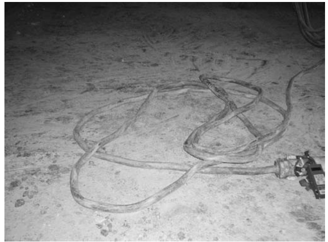
Figure 3a — Shredder cable haphazardly overlapped.
