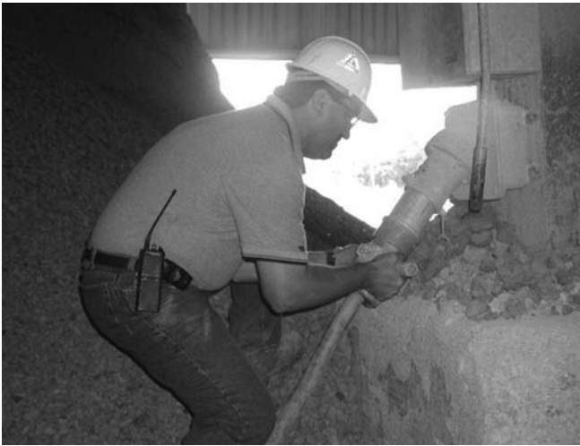
Figure 1 — Mineworker demonstrates power connection.
