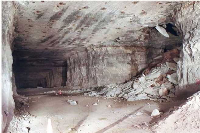
Fig. 2. Roof failure at Case Study 1, view looking down dip.
