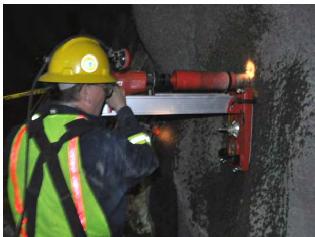
Figure 64. Wet drilling a 102-mm (4-in) diameter hole for the shotcrete adhesion test core (note bit change).
