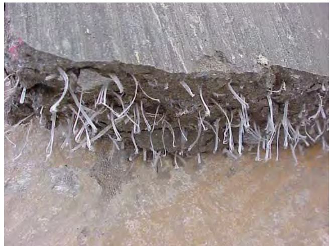
Figure 79. Synthetic macro fibers exposed along the failure surface of round-panel shotcrete sample.
