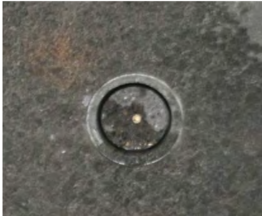
Figure 67. Adhesion test #2: core broke entirely in the top layer of shotcrete.
