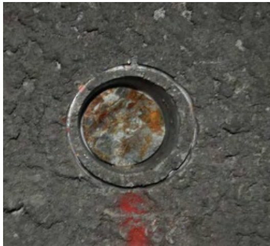
Figure 68. Adhesion test #3: core broke prematurely in weak underlying host rock.
