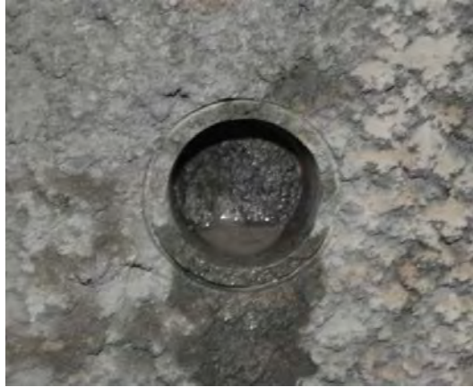
Figure 66. Adhesion test #1: core broke in shotcrete and at interface between two shotcrete layers.
