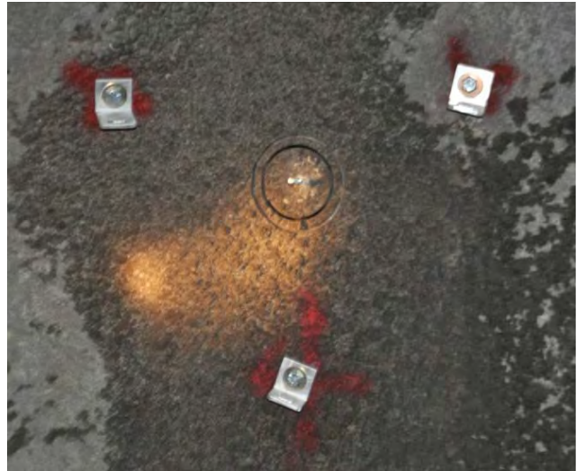
Figure 58. Strap brackets centered around the epoxied stud to anchor the direct-tension test equipment.
