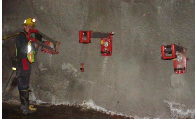
Figure 62. Shotcrete adhesion test site with three drill stands mounted on mine rib.
