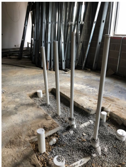
Figure B4. Plumbing work in the renovation area completed overnight before the reported incident. Photo by NIOSH.
