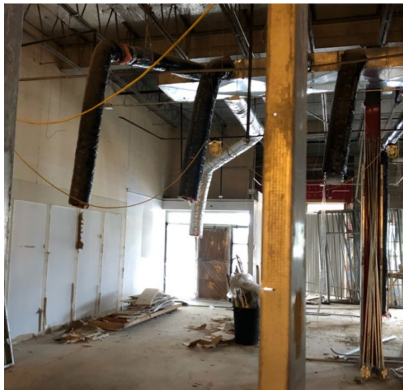
Figure B3. Renovation area showing sealed door (back), which was the main entrance to the area, and a sheet rock wall, which was part of the hallway across from Agency A offices. Photo by NIOSH.
