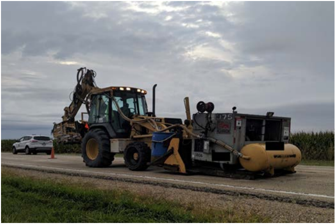
Figure A1. The entire backhoe and drill rig setup. The drills are mounted on the arm of the backhoe and the water control system is mounted on the front. The water control system is connected to the drills with tubing. Photo by the National Institute for Occupational Safety and Health (NIOSH).
