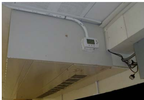
Figure B2. Typical classroom ceiling-mounted unit ventilator. Photo by NIOSH.
