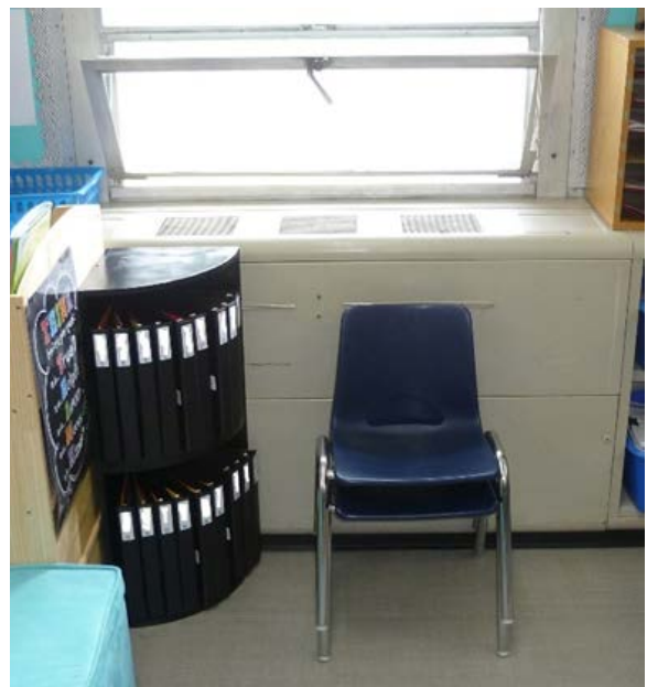
Figure 1. A classroom unit ventilator is partially blocked by furniture and classroom supplies. The window above it is open. Photo by NIOSH.
