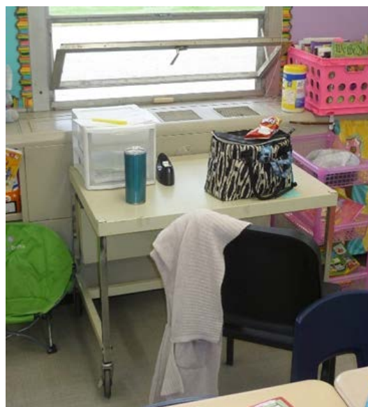
Figure B1. A typical classroom unit ventilator. Photo by NIOSH.
