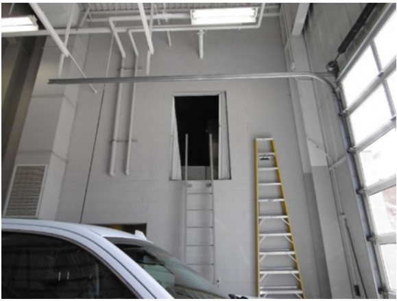
Figure 4. Ladder and opening to the mechanical room containing the three air handling units that supplied air to the living quarters.
