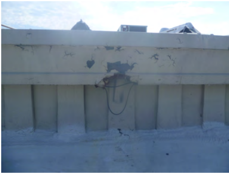
Figure 2. Gutter with a large hole rusted through. Photo by NIOSH.
