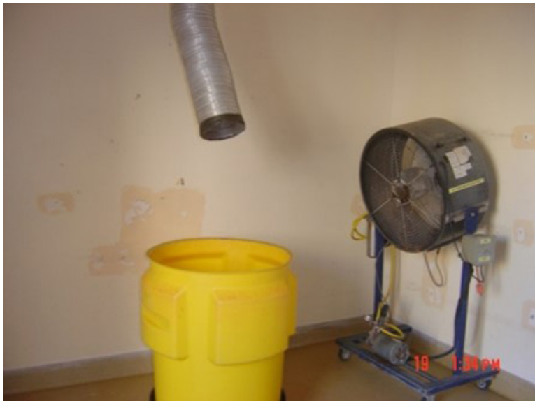
Figure 6. Tray scraping operation area prior to installation of the LEV hood. Photo by NIOSH.
