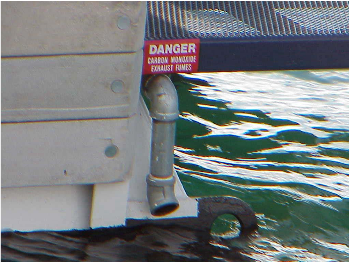
Figure 3. Generator exhaust discharge on the Grand Sierra Pontoon Houseboat.
