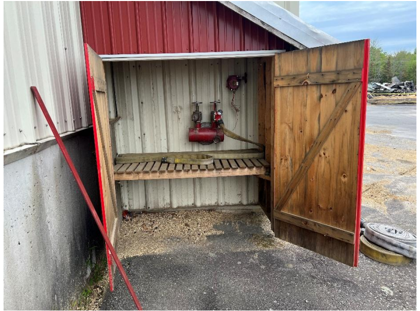
Image 4. Station containing hoseline for facility fire suppression, post-incident. (Source: NIOSH)
