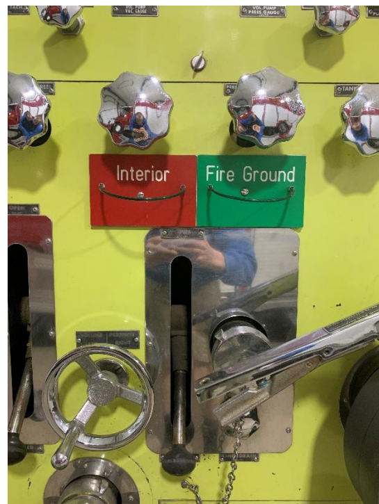
Image 14. Accountability rings on pump panel. (Source: Fire department)
