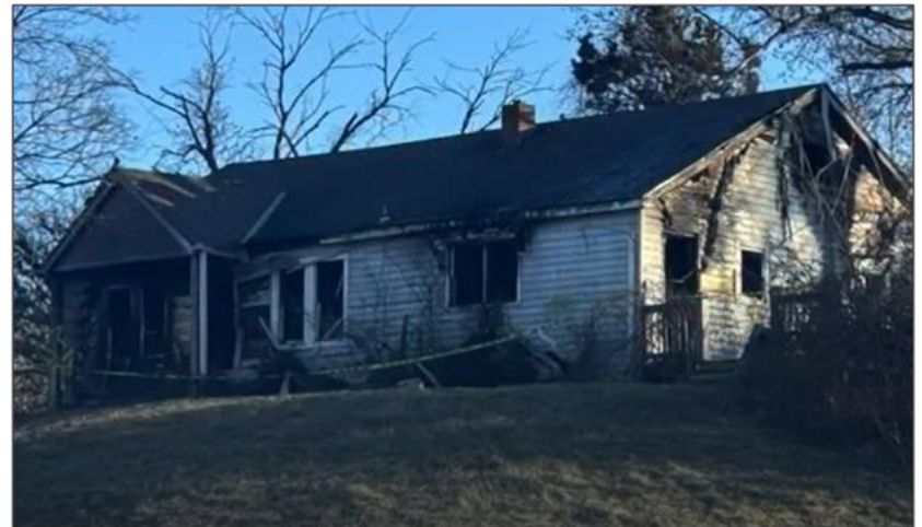
View of Side Alpha of structure, post-fire. (Courtesy of the fire department)
