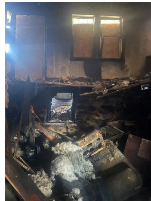
View of area of collapse with debris. (Courtesy of the fire department)
