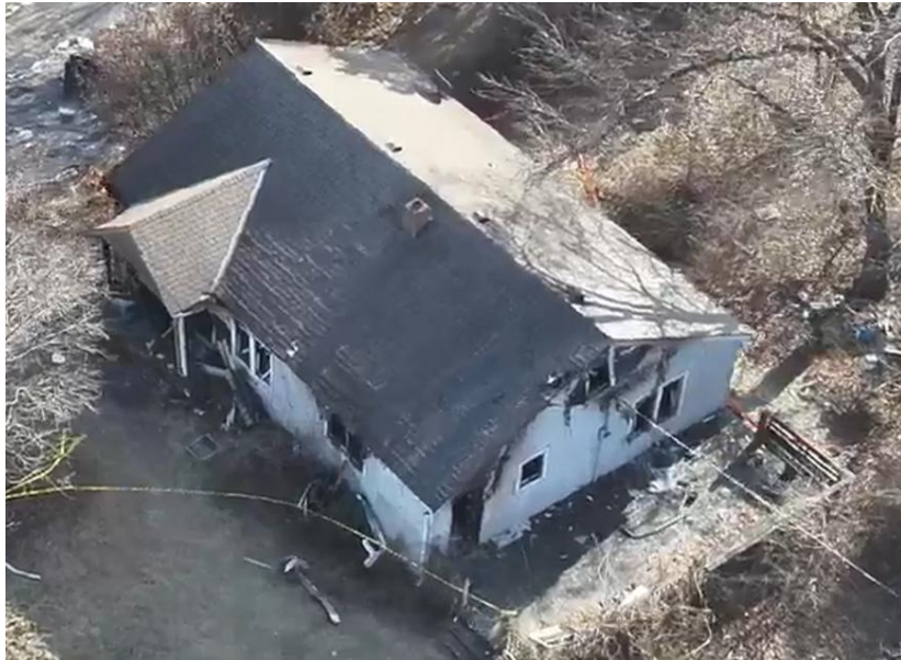
Aerial view of structure, post-fire. (Courtesy of the fire department)
