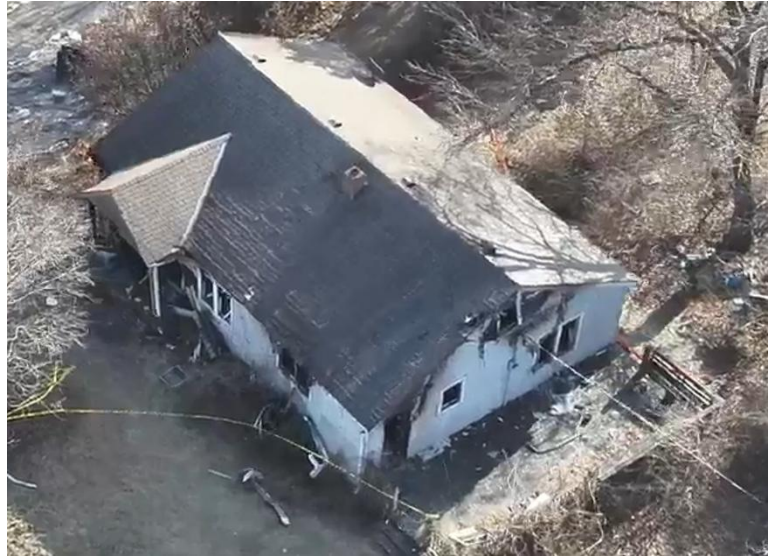
Photo 2: Aerial view of structure, post-fire. (Courtesy of the fire department)
