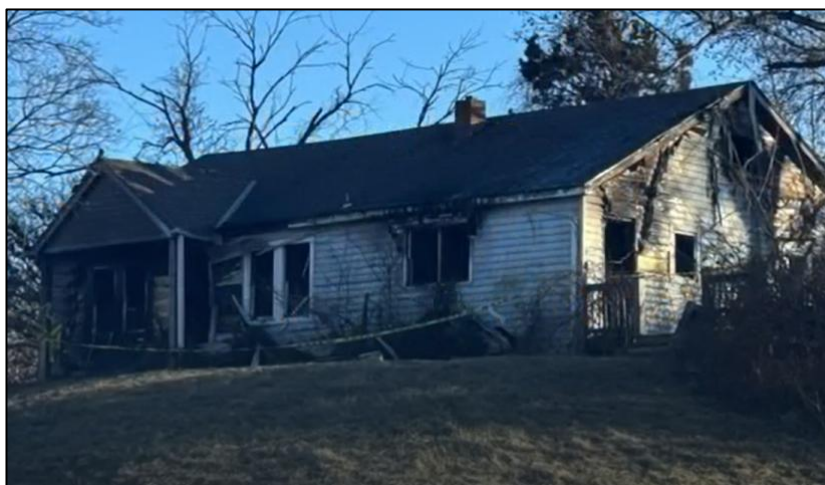
Photo 1: View of Side Alpha of structure, post-fire. (Courtesy of the fire department)
