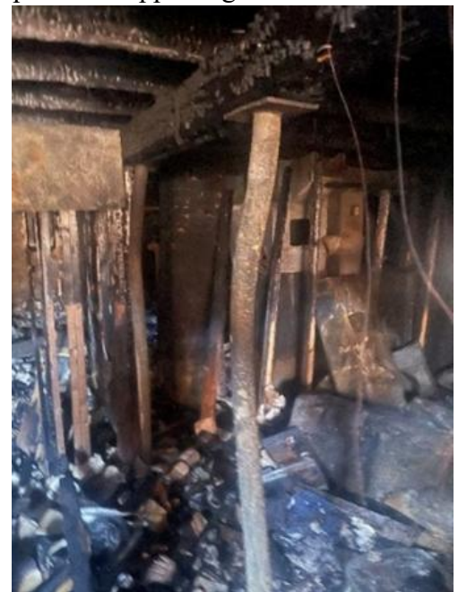
Photo 7: Twisting of steel column. (Courtesy of the fire department)
