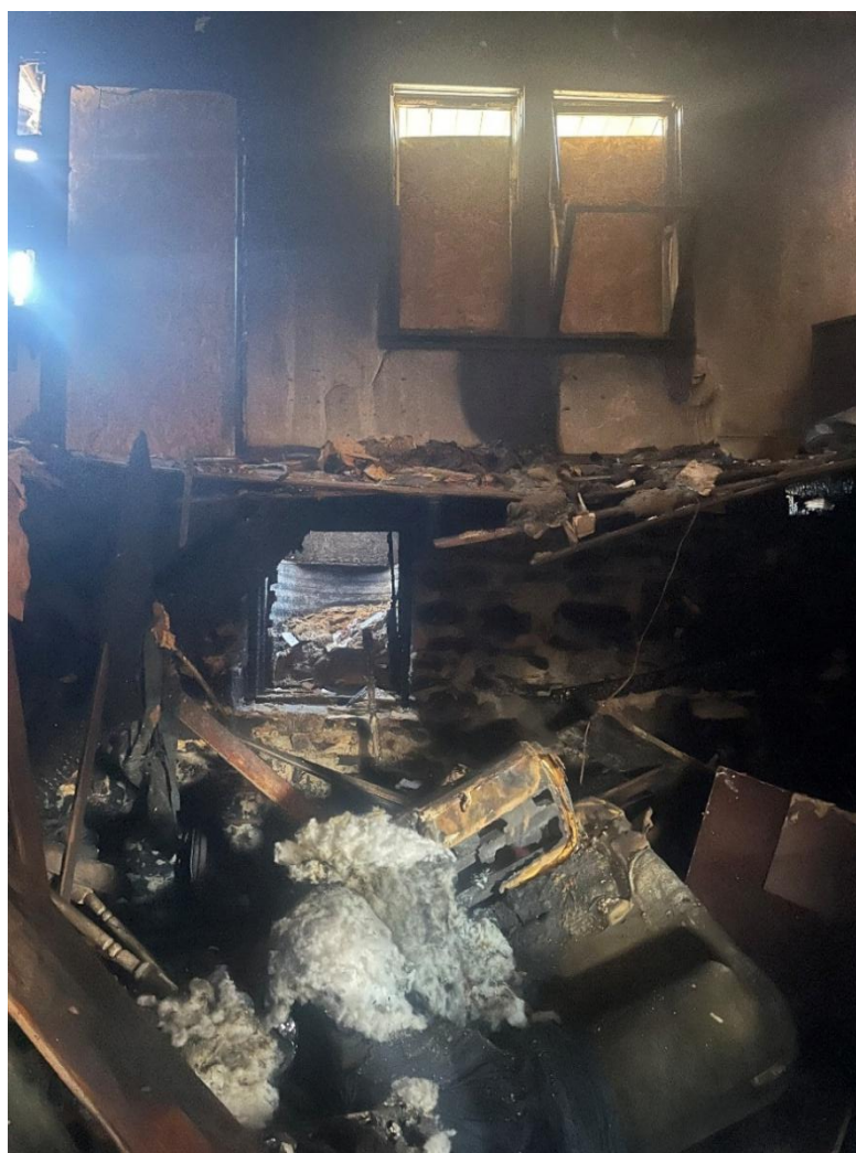
Photo 11: View of area of collapse with debris. (Courtesy of the fire department)
