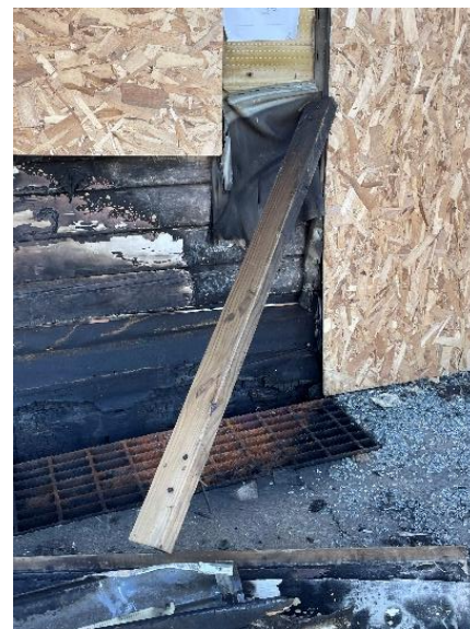
Photo 9: Grate cover over basement window. (Courtesy of the fire department)
