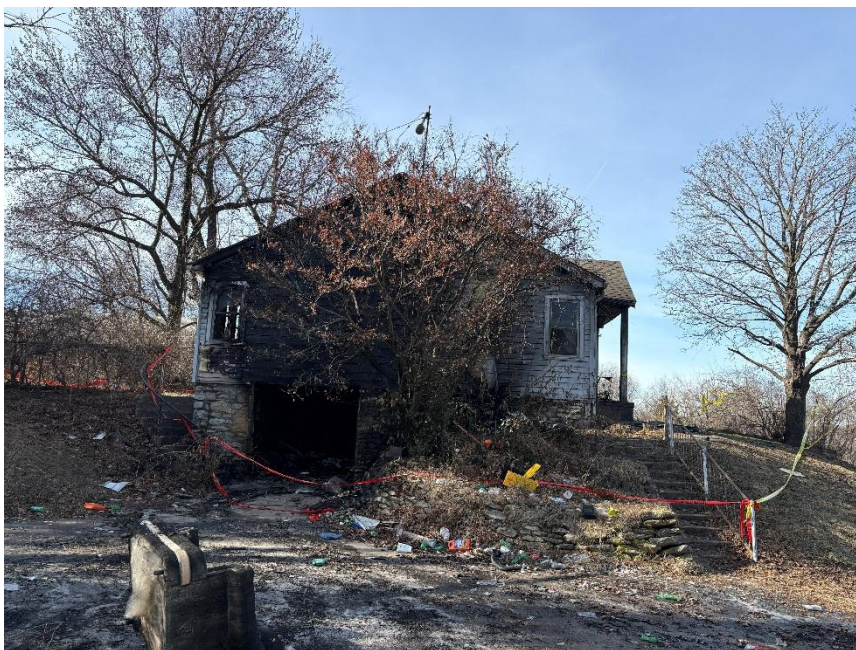
Photo 8: View of Side Bravo garage entrance, post-fire. (Courtesy of the fire department)
