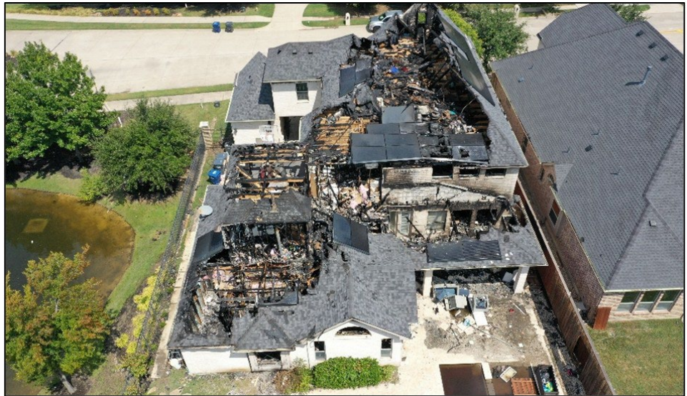
View of the rear of structure, post-fire. Photo courtesy of the fire department.
