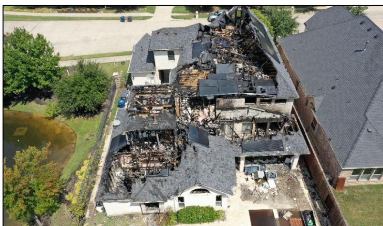
Photo 1: View of the rear of structure, post-fire. (Courtesy of the fire department)
