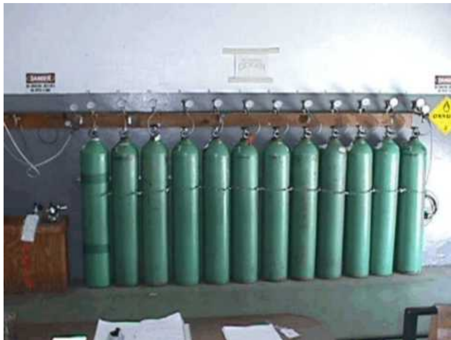
Photo 4: This photo depicts the cascade system used by the fire department to refill the oxygen cylinders. The cascade system is composed of 12 M-size (300 cubic
