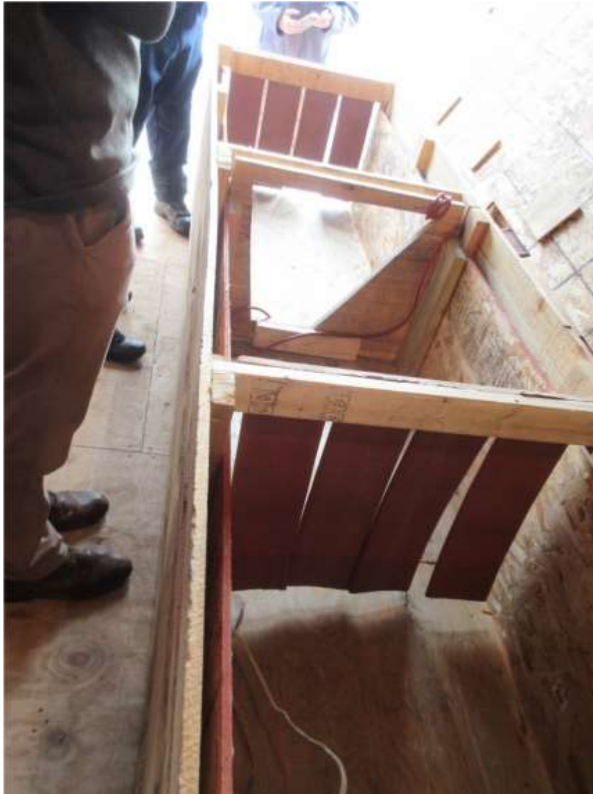
Photo 2: Third restricted opening in the tunnel prop (Photo by NIOSH)
