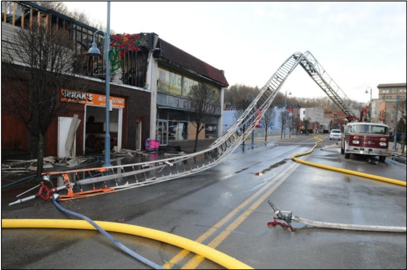
Photo 5. Note 5-inch supply hose laid from one side of the street to the other causing the driver of the aerial apparatus to stop short of fire structure. (NIOSH Photo)
