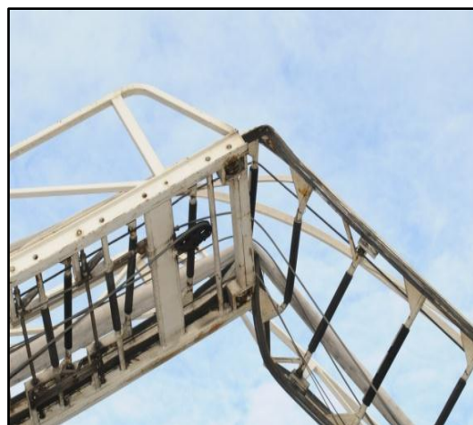
Photo 6. Structural failure occurred at end of the ladder bed section. (Courtesy of the Fire Department)
