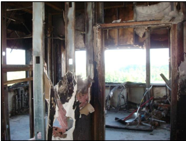
Photo 2. Fire room at A/B corner of structure. View from the end of Side A hallway. (NIOSH photo)
