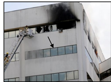
Area of fire origin – A/B corner (Courtesy of Fire Department)
