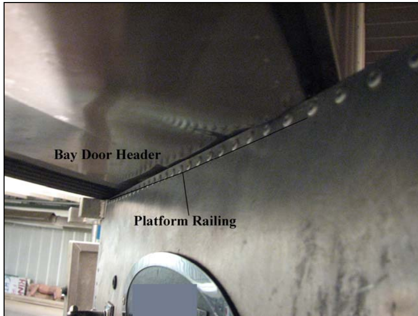
Photo 9. The level of clearance observed between door header and platform railing. (Photo courtesy of consultant group during reconstruction of the incident.)
