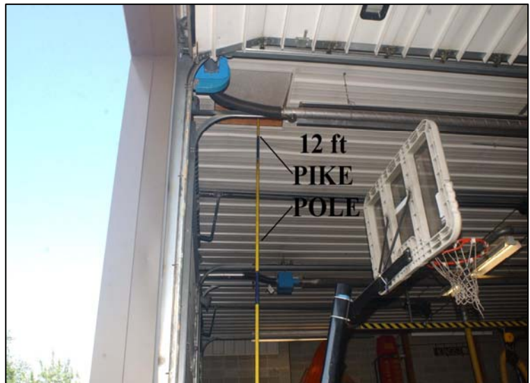
Photo 5. Pike pole stuck in scuttle hatch. (Photo courtesy of police department.)
