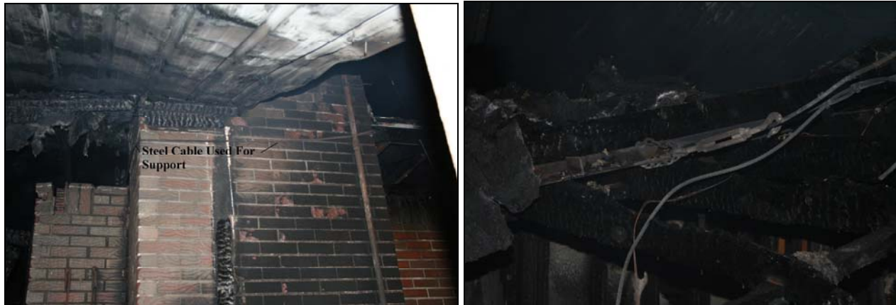
Photo 1. Steel cable used to support the chimney against the house with a turnbuckle. (Photos courtesy of sheriff's office)
