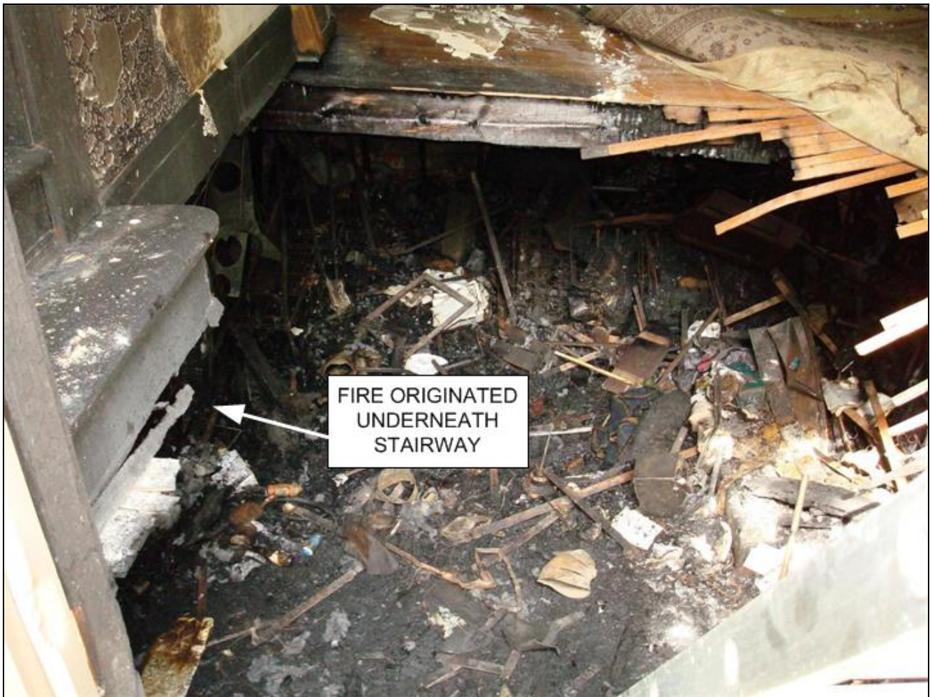
Photo 4. View of fire structure's floor collapse just inside the B-side french door. The fire originated underneath the step shown on the left. (NIOSH Photo)
