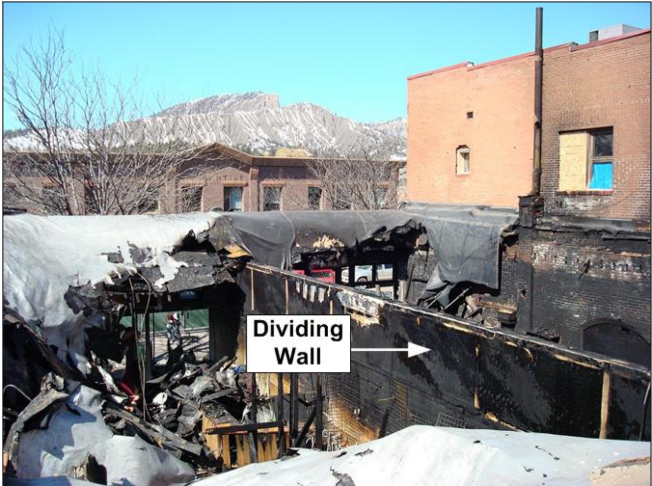
Photo 2. This picture shows the restaurant (fire structure) on the right and the involved adjacent retail store on the left (exposure D1) (see Diagram 1). The building had been remodeled several times which included dividing the building in half via a wood stud wall (in middle of photo), lowering the ceiling in both halves yet sharing a common attic space. (NIOSH photo)
