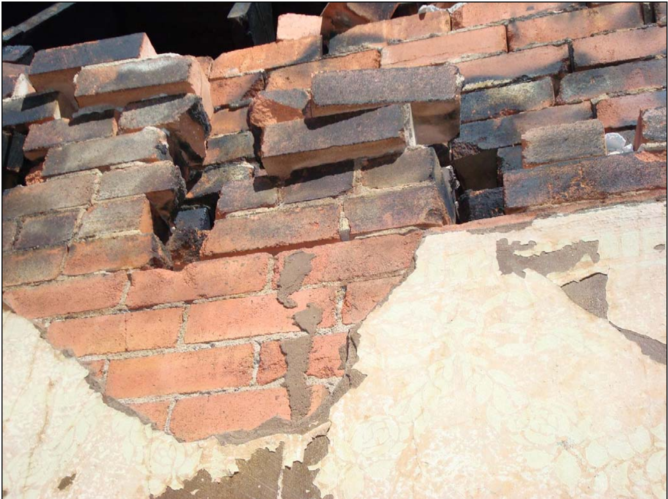
Photo 4. Exposure D2's B-side wall with existing 2" x 4" holes in the void space area. (NIOSH photo)
