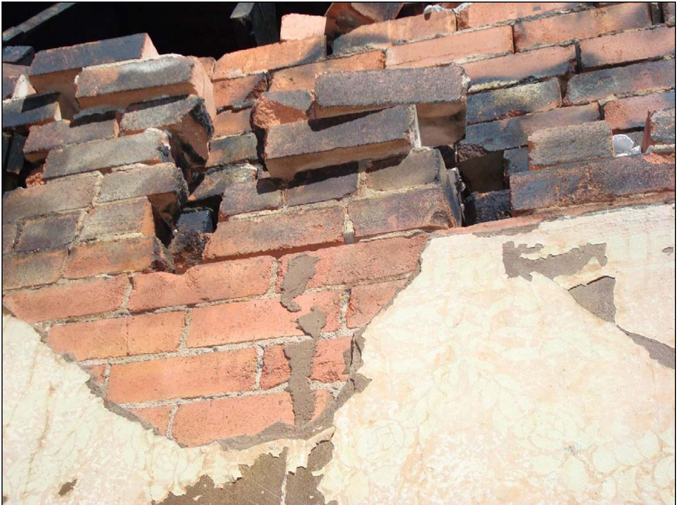
Photo 4. Exposure D2's B-side wall with existing 2" x 4" holes in the void space area. (NIOSH photo)
