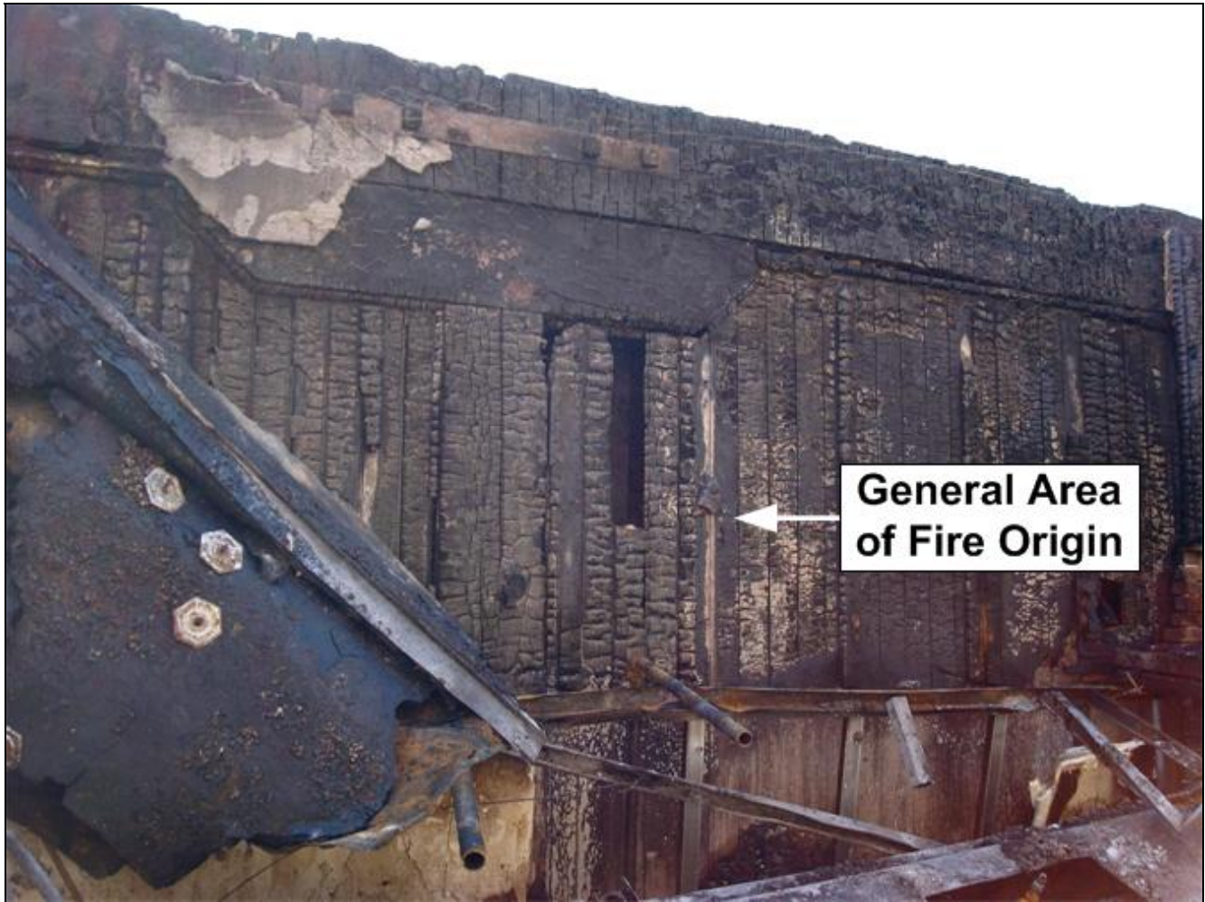
Photo 3. The fire structure's D-side wall where the fire originated in the duct work above the wood grill. (NIOSH photo)
