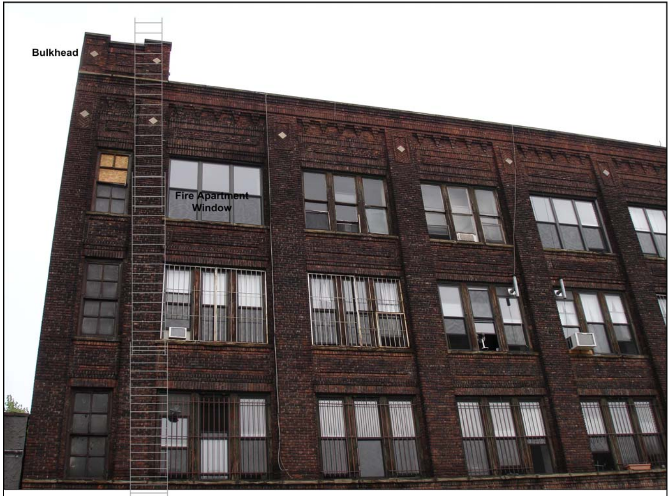
Photo 1. Incident Structure. (Ladder image is for reference purposes only) (NIOSH photo)
