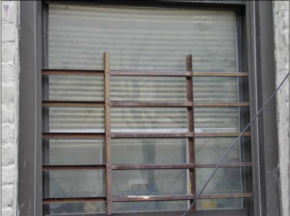
Photo 3. Child Guard Gate on Apartment Windows
