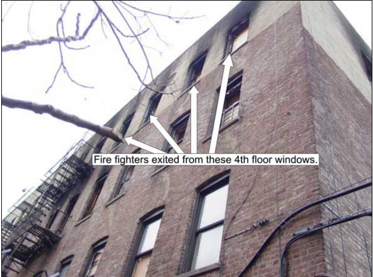
Photo 2. Rear of Incident Structure
