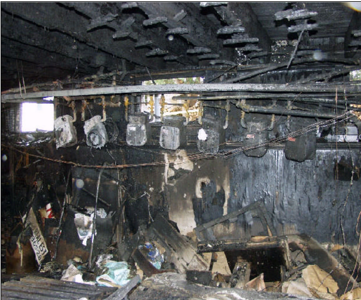
Photo 3. The two compromised gas meters are on the left.
