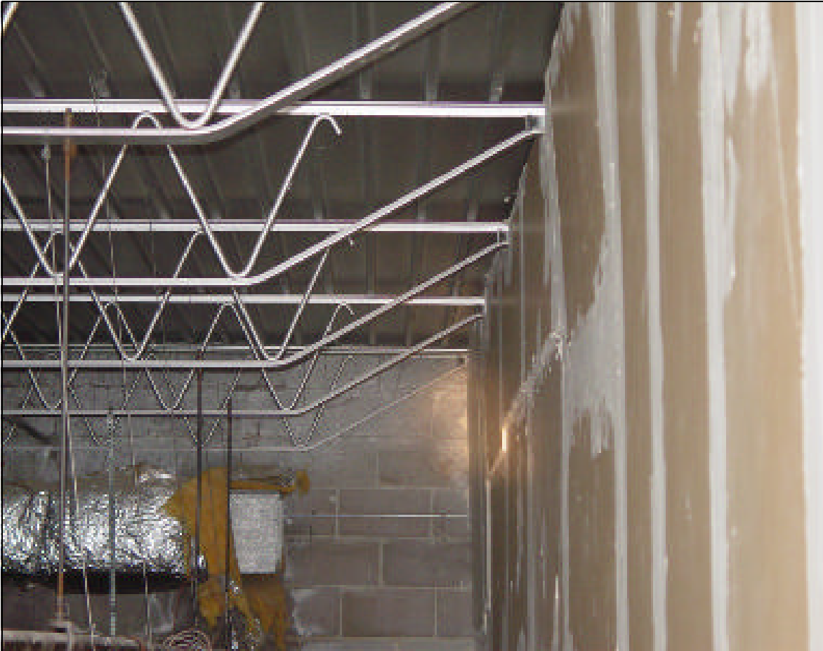
Photo 1. Void space between the corrugated metal roof sheeting and suspended ceiling where the unprotected open-web steel trusses are located. This photo was taken from a building similar in construction to the building involved in this incident.
