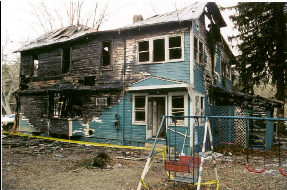
Photo 2. Rear of incident structure
