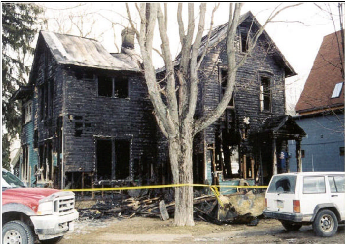
Photo 1. Front of incident structure
