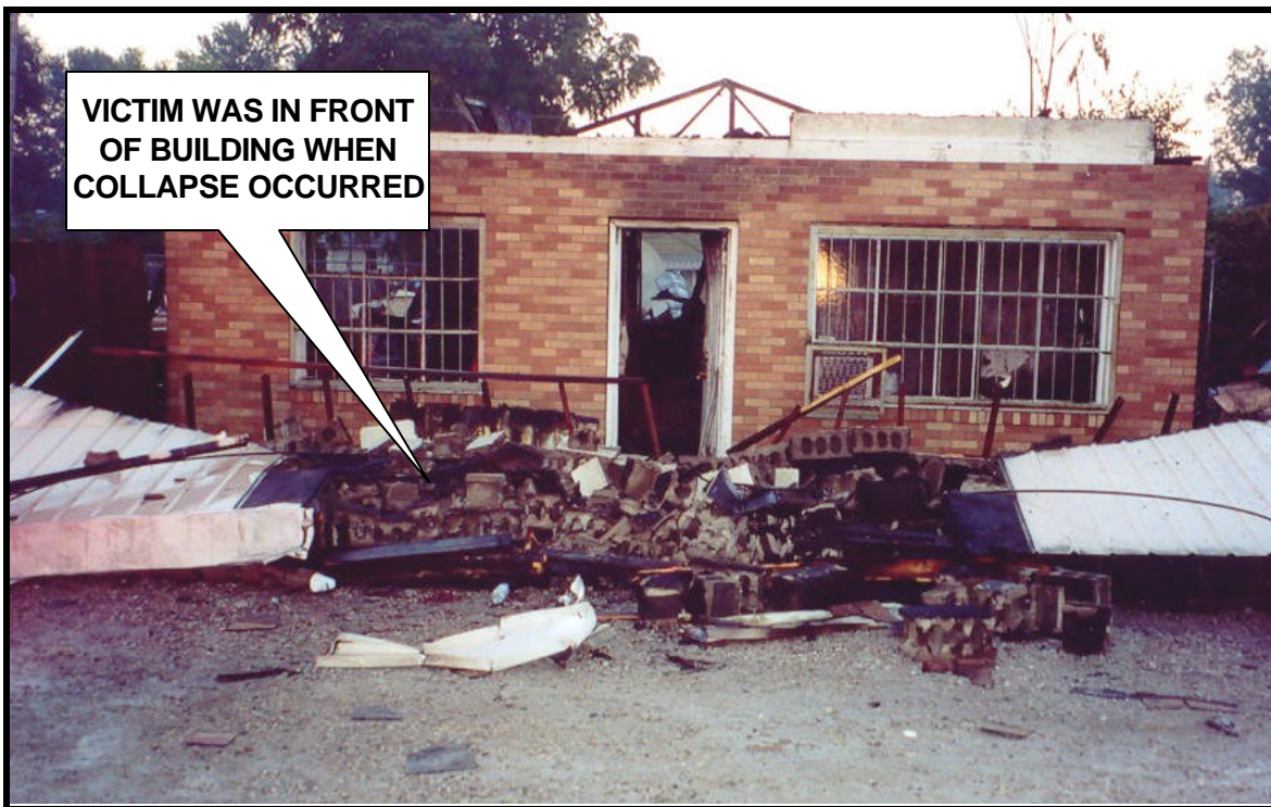
Photo 3. A-side of building after collapse
