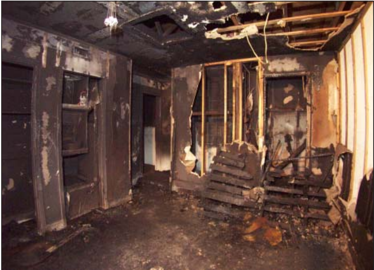
Photo 2. Burn room in the structure
