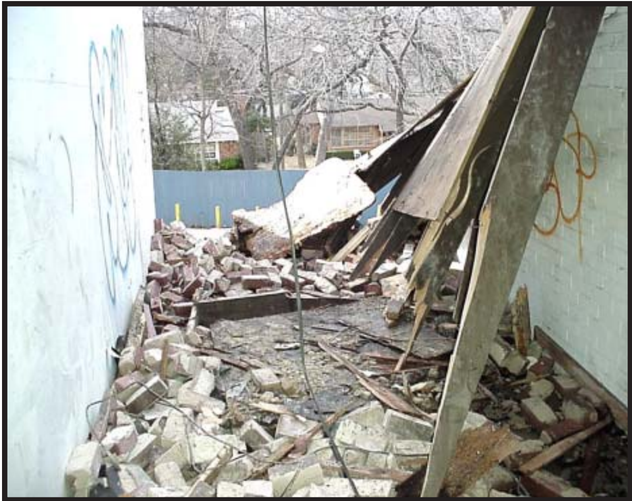
Photo 1. Area of Collapse
