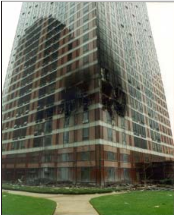
Building Involved in Fire
