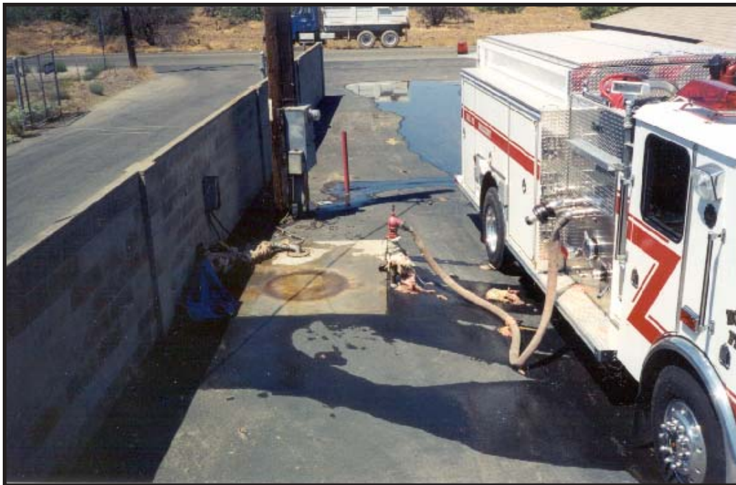
Photo 3. Illustrates the original placement of the water holding tank, the hydrant, and the plumbing system in relation to the passenger side of the engine.
