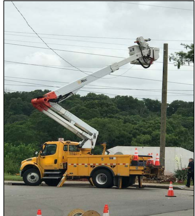
Position of bucket truck in cul-de-sac at the time of the incident. (Photo courtesy of the City)
