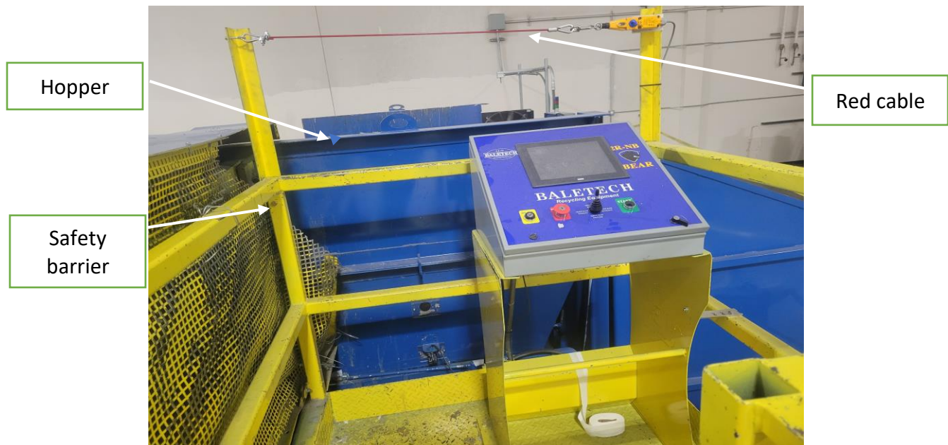
Exhibit 6. The yellow barrier around the control panel to prevent access to the hopper. The red cable was added after the incident occurred. Photo by CA/FACE program.
