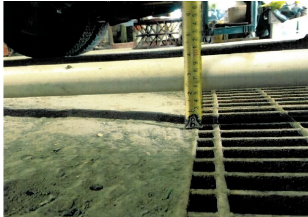
Photo 6: Floor gradient at Bay 1 central drain over 10-foot span (phot courtesy of PESH)
