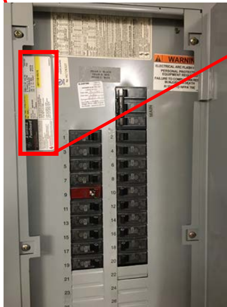
Image 3. 208/120V electrical panel controlling accent lighting and store outlets, with close-up of information sticker on inside of the breaker panel box. Note this is a 3-phase panel.
