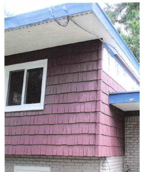
Photo 2. Lower level and upper level roof. Area of home where siding was to be installed and where decedent was working.
