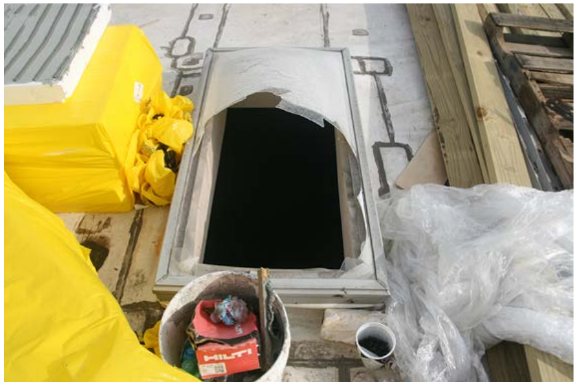
Photo 6. Skylight involved in incident
