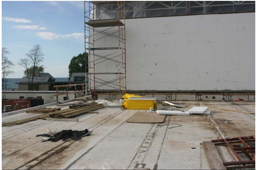
Photo 4. Incident area, looking north
